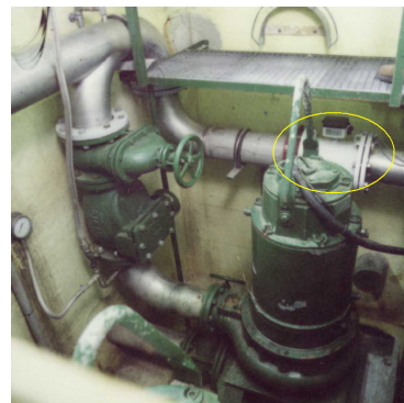
A DN200 MAG-meter (yellow circle) installed in a well very close to tube bends, valves and a pump
